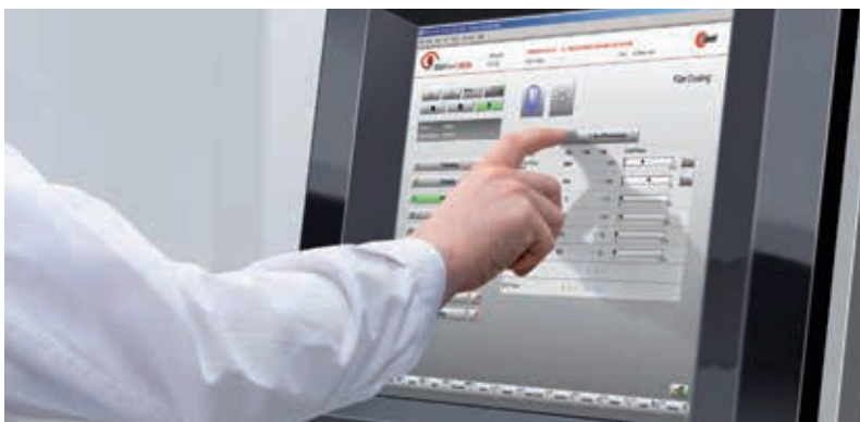
Control system including operating and data management
