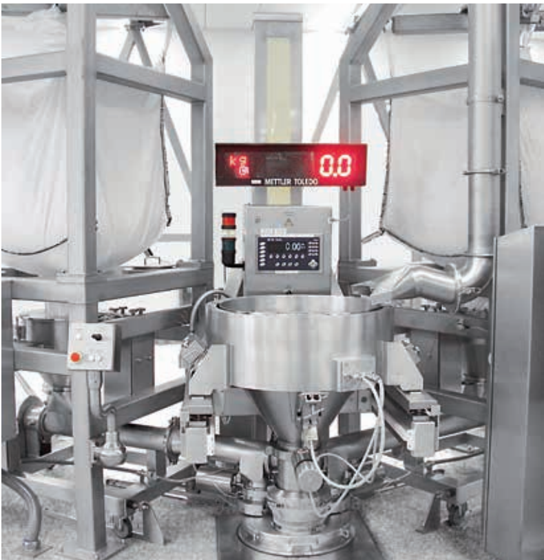
Combined raw material dispensing from big-bags and sacks into ICBs
